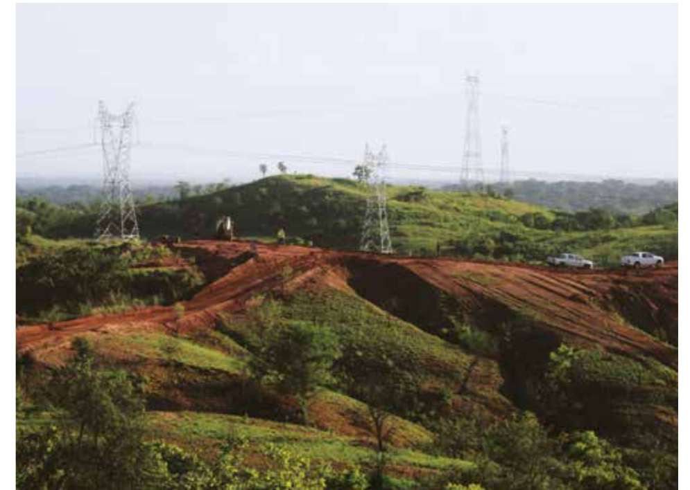
↑ 400 KV Laúca-Bita Transmission Lines - Section II, Angola
