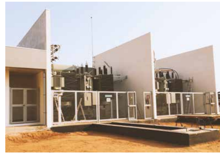
↑ Chicala Substation Chicala, Luanda, Angola
