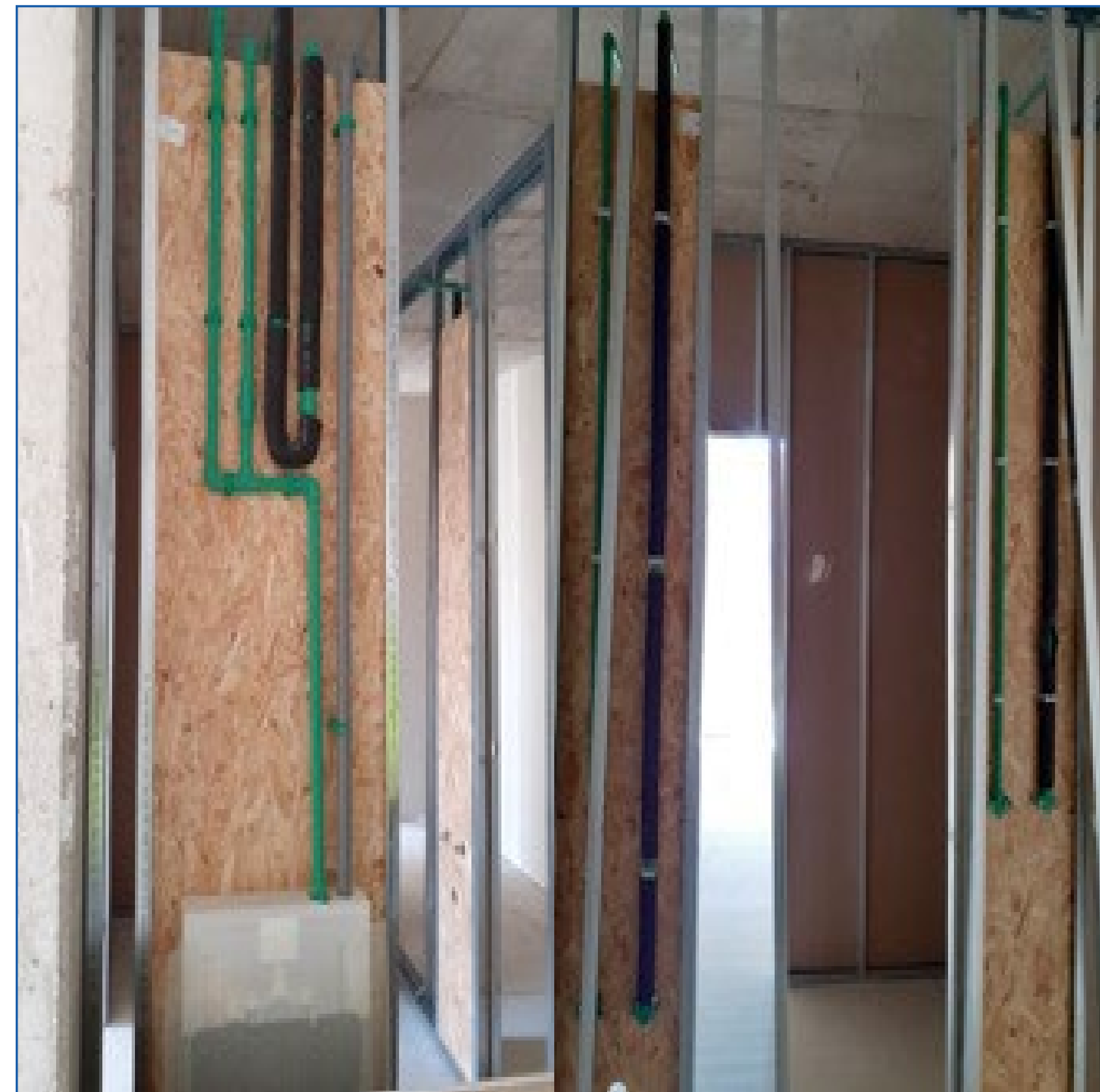
Fig.3 -Hydraulic infrastructure plates on the infrastructure walls on site
