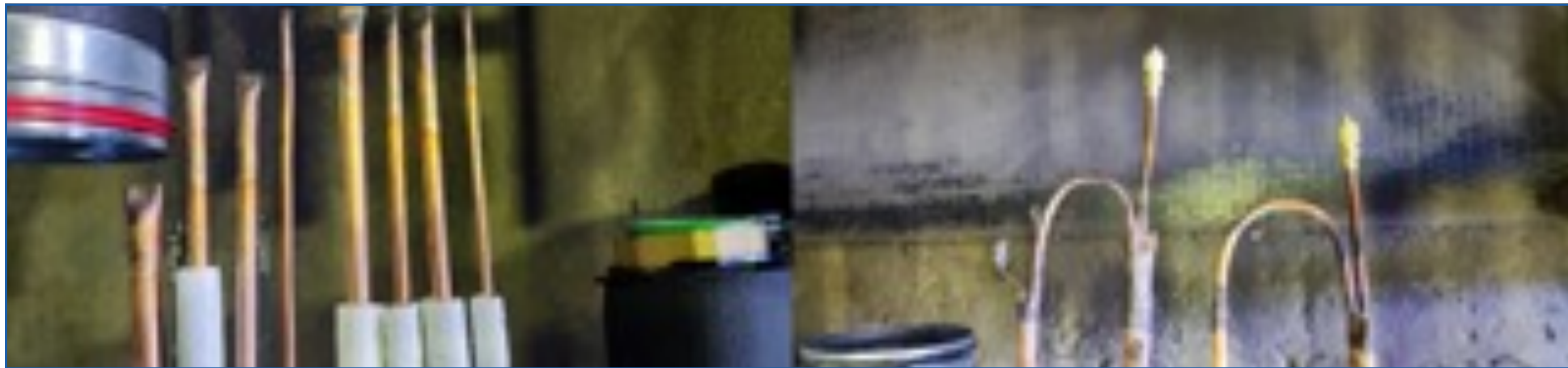
Fig.12 - Insulated copper piping pressurized with Nitrogen at 41 bar, so that the welder responsible for the joints on site is aware of the occurrence of leaks, during transport or assembly of the modules. Long and laborious process.
