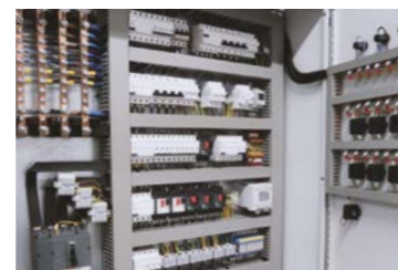
Quadrina Typified Electrical Boards
